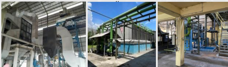
Palembang, Sumatera Selatan Factory, Rice Husk-fueled Power Plant with Capacity of 3MW
